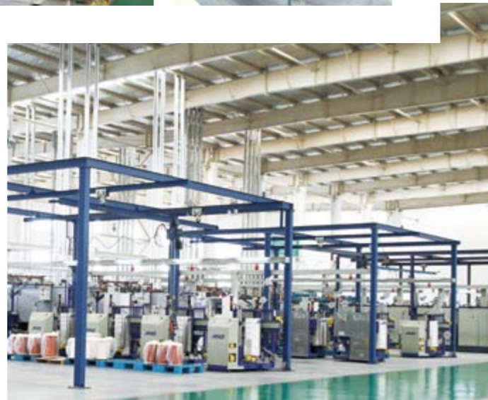
MAG Plant MAG生产车间
